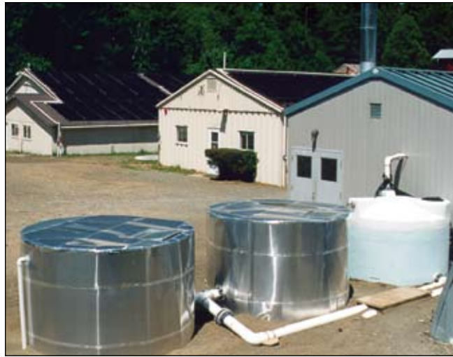
Figure 5: Solar Water Heating Project at a Salmon Hatchery, Canada.
