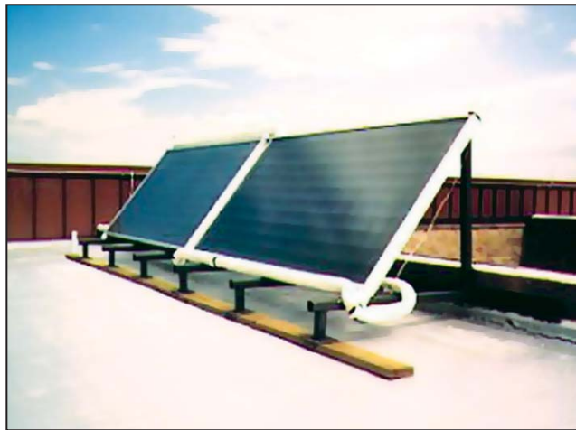
Figure 10: Solar Water Heating System.
