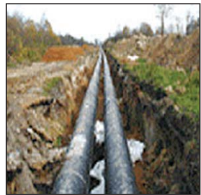
Figure 3: Water Pipes in District Heating System.
