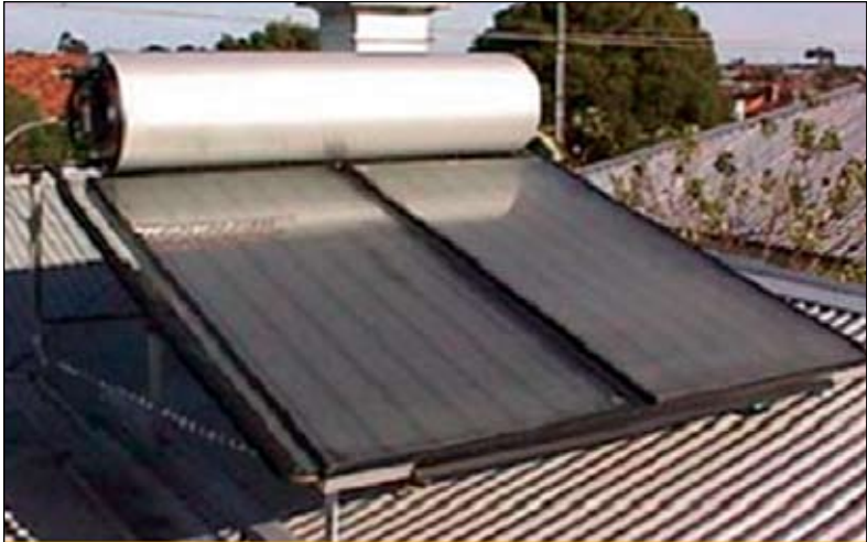
Figure 2: Solar Domestic Hot Water (Thermosiphon) System in Australia.
