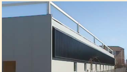
Solar Air Heating Technology, Yellowknife, NWT, Canada.
