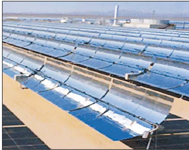
Figure 18: Parabolic-Trough Solar Power Plant.
